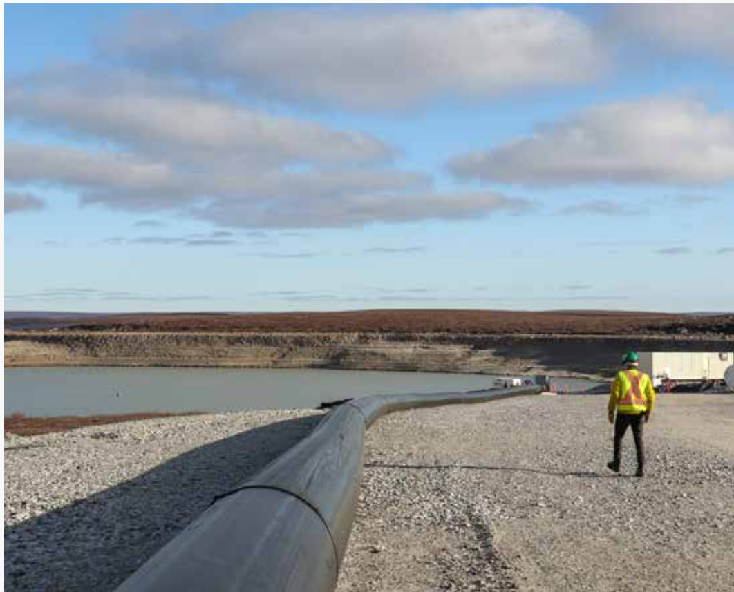
Dewatering pipe along Point Lake Road - 2022 site visit
