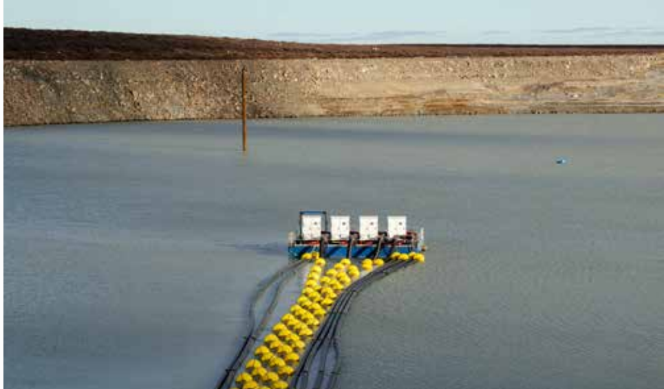
Point Lake dewatering pumps - 2022 site visit
