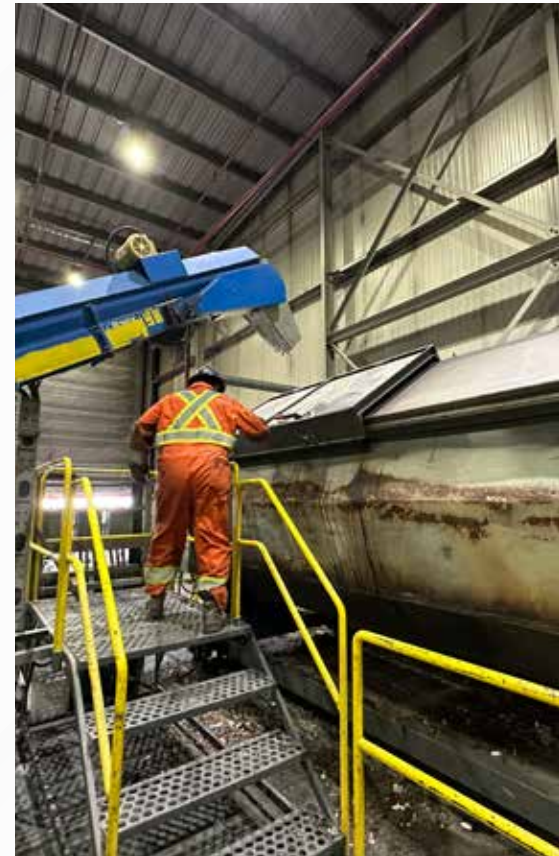
Opening composter at incinerator composter building
