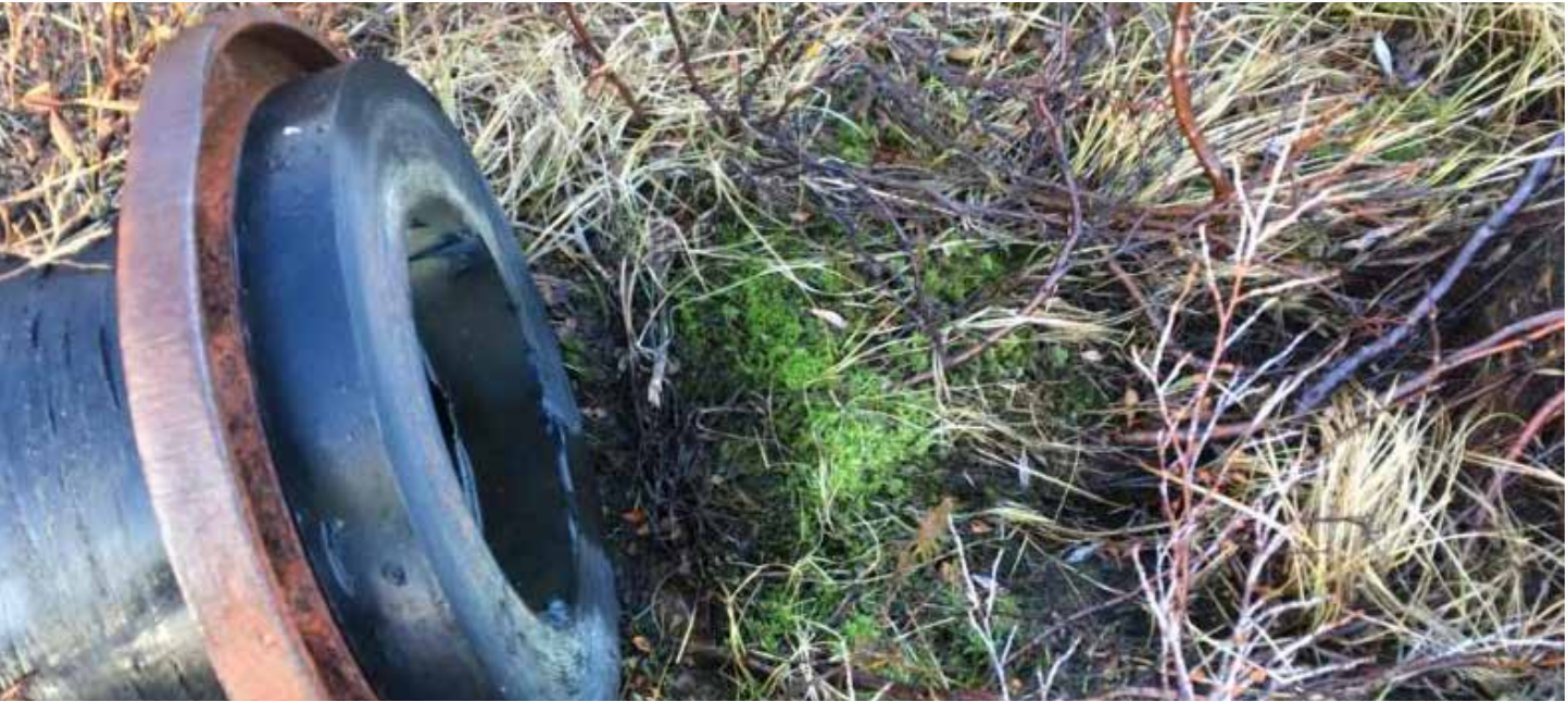
Effluent 'discharge' pipe to Horseshoe Lake.
