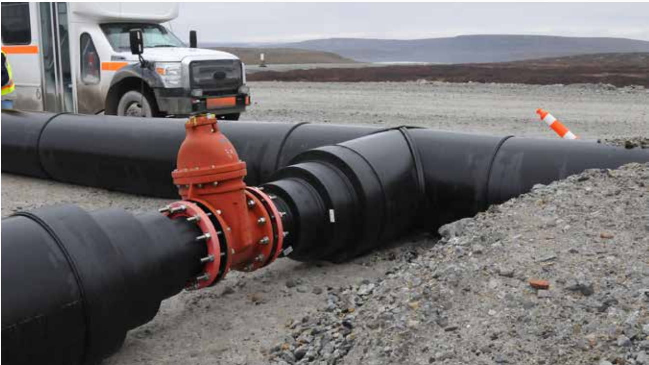
Large diameter insulated pipe for moving water and processed kimberlite on site, photo taken during site visit 2024.
