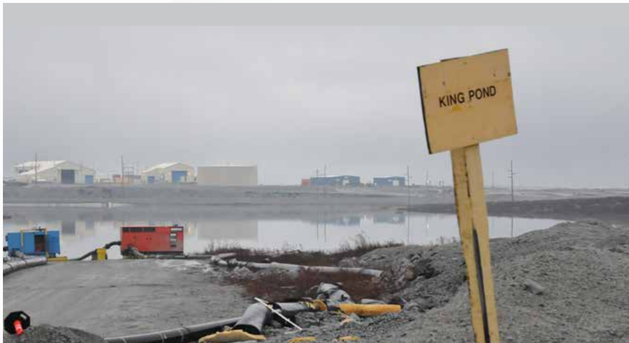
Insulated pipe in disrepair and insulation blowing around by King Pond Settling Facility 2023.
