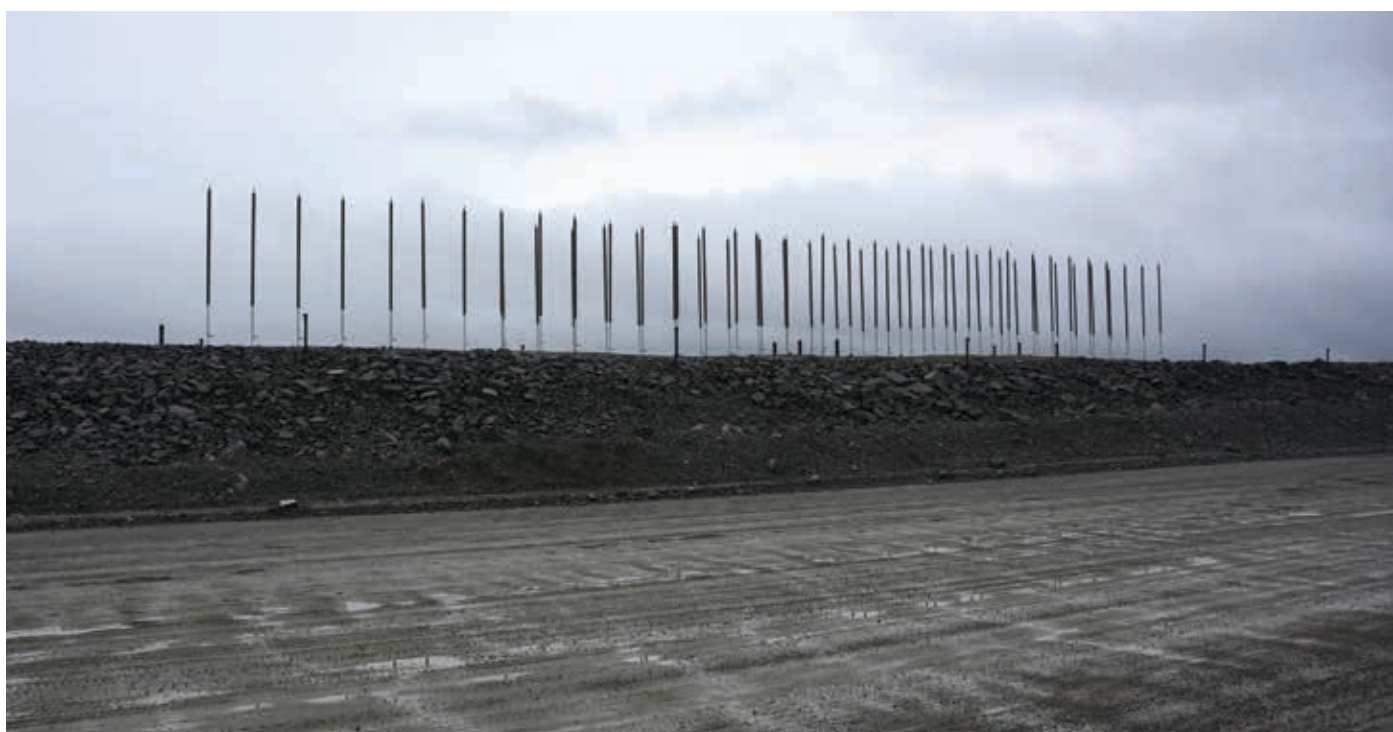
Thermosiphons at the compliance point of discharge for the Long Lake Containment Facility, October 2023
