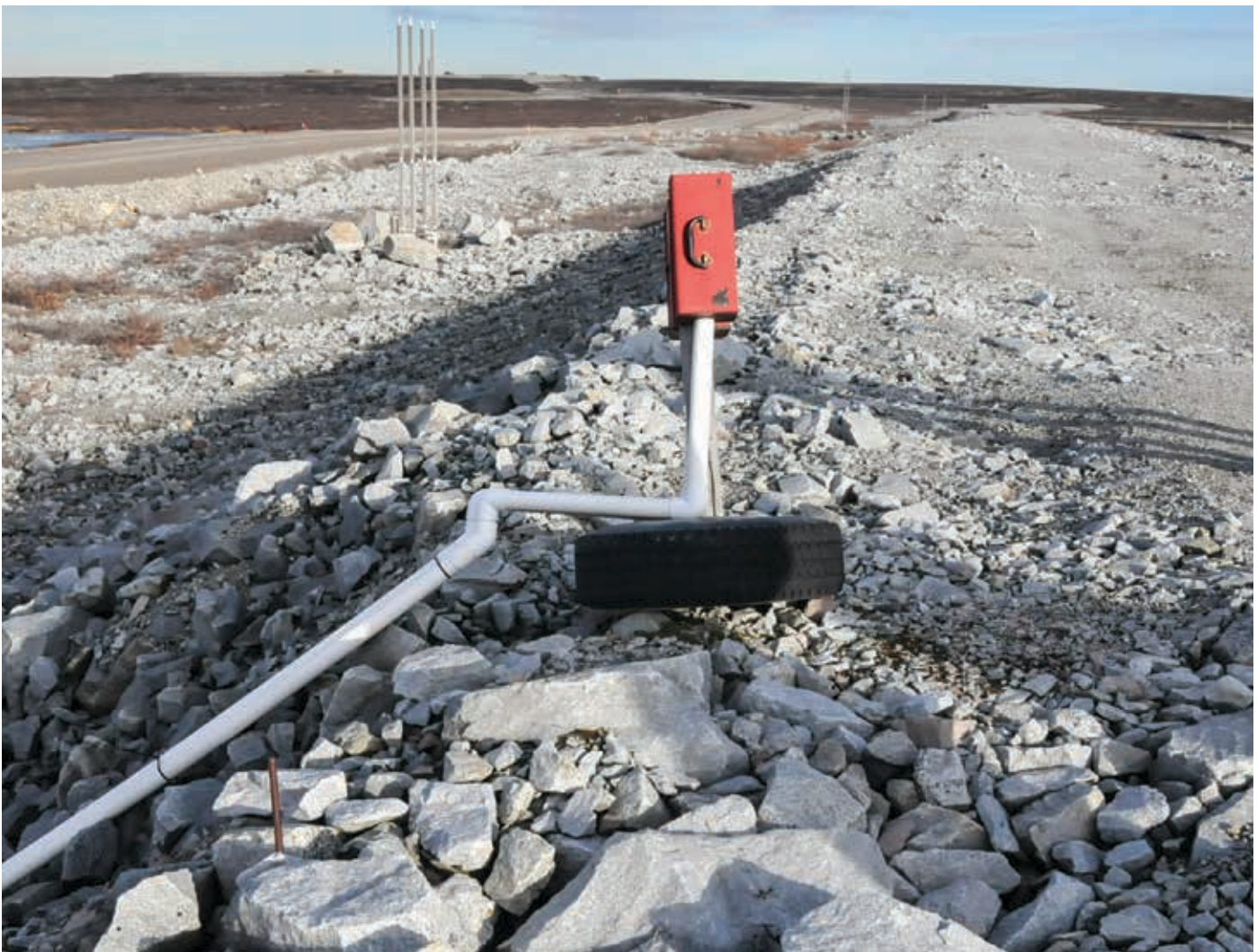
Thermister cable access near Cujo Lake, October 2024
